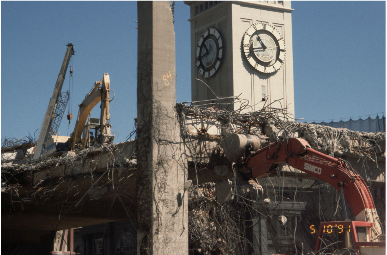
Construction crews tear down the Embarcadero Freeway, with the Ferry Building towering in the background.
